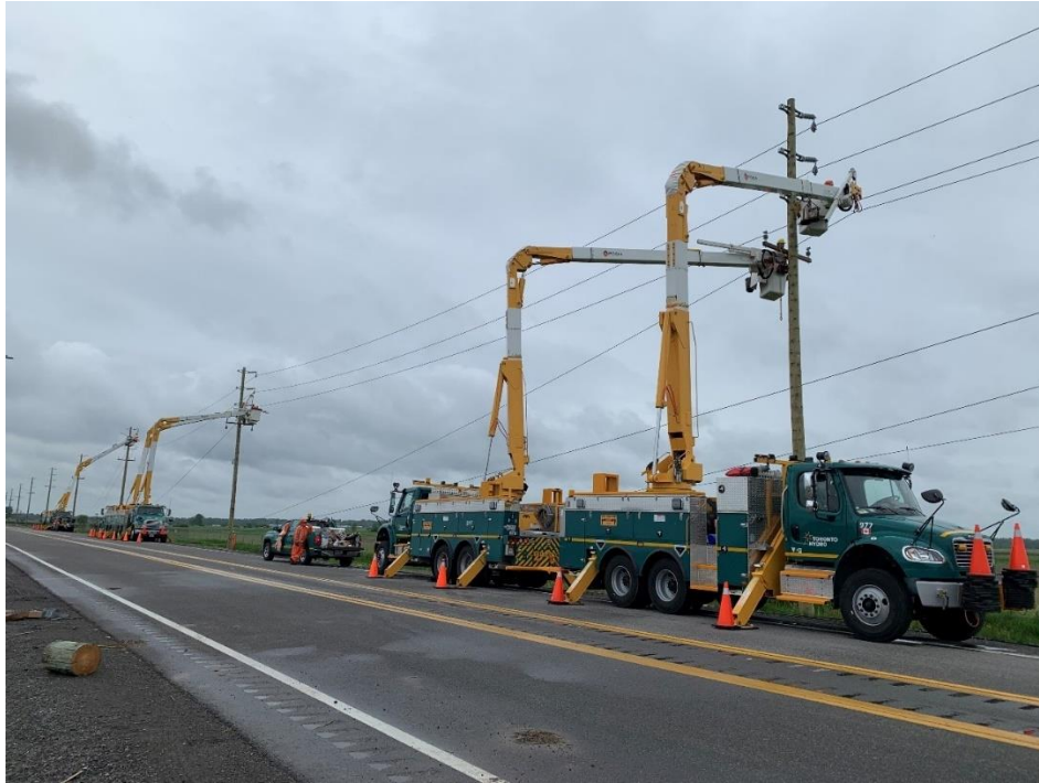
4 Figure 4: Repair Work by Toronto Hydro Crews Deployed to Hydro Ottawa Territory 5 (May 2022)
