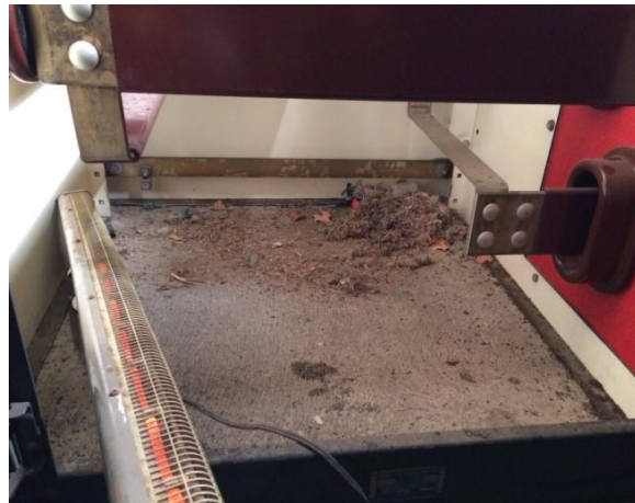
Figure 16: Pests Inside Outdoor Switchgear
