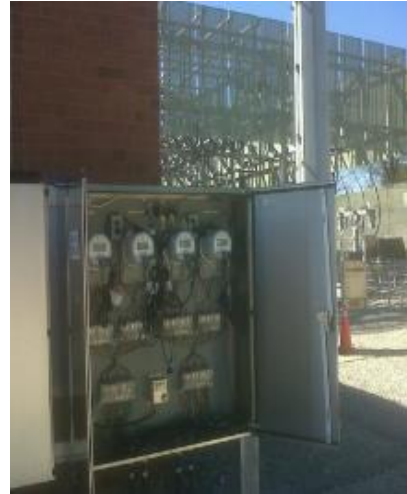
Figure 18: Wholesale Meter Installation at Transformer Station.
