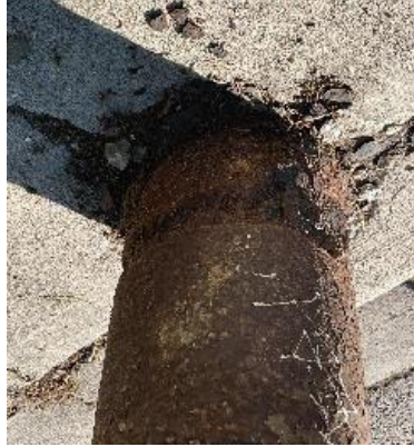
4 Figure 5: Corrosion on Steel Pole Base
