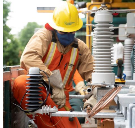
PLT - Overhead Plant
