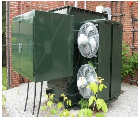
11 Figure 20: Power Transformer at Neilson Dr. MS
