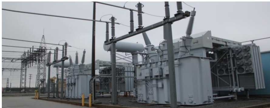
Figure 8: The Station Yard at Cavanagh TS
