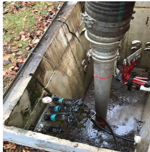
Figure 9: Crews Cleaning a Vault that had a Transformer Oil Leak
