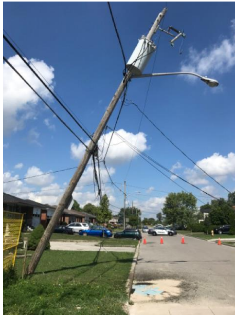
5 Figure 6: shows a leaning distribution pole Grid Response crews attended to and 6 forwarded for permanent reactive repair (2021)
