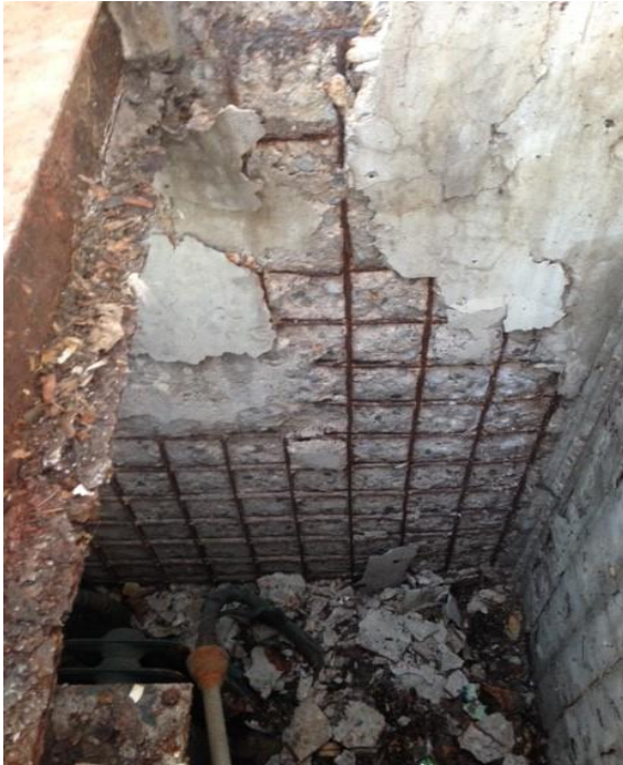
Figure 3: Crumbling Vault Roof with Exposed Rebar
