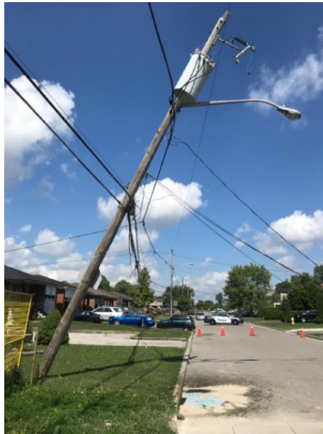
5 Figure 6: shows a leaning distribution pole Grid Response crews attended to and 6 forwarded for permanent reactive repair (2021)
