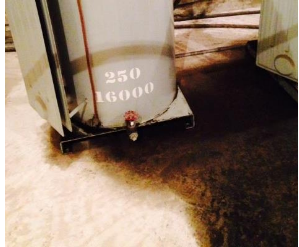
Figure 3: Transformer Leaking Oil
