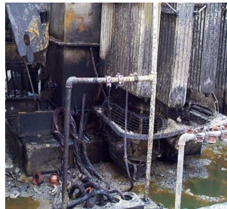
Figure 24: Leaking Fluids from Failed Transformer
