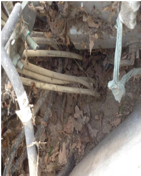
Figure 6: Vault Full of Dirt and Debris
