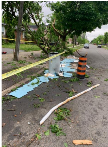
10 Figure 7: shows an Overhead Transformer taken down by a falling tree, spilling oil 11 onto the roadway and sidewalk (2022)
