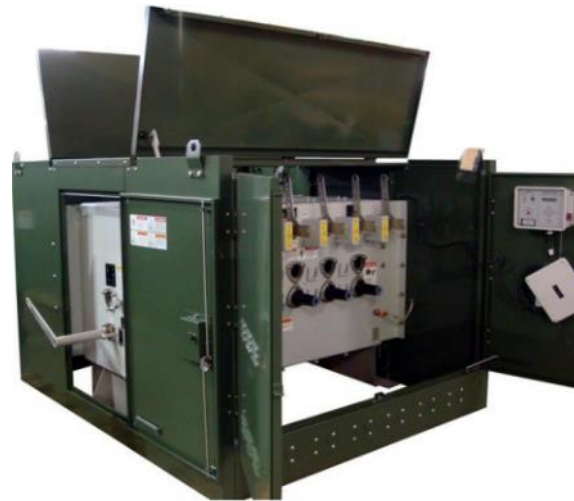
Figure 12: Padmounted SF6-Insulated Switch
