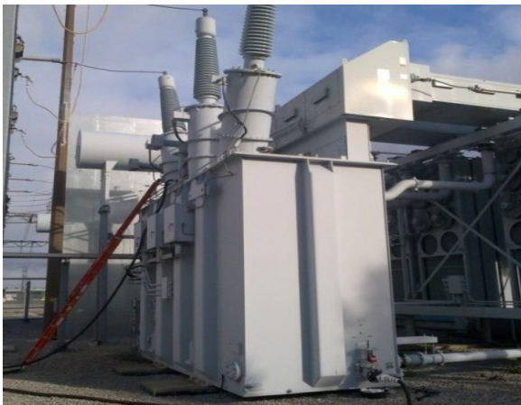
9 10 Figure 19: Power Transformer at Cavanagh TS
