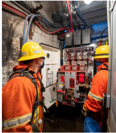
PLT - Underground Plant
