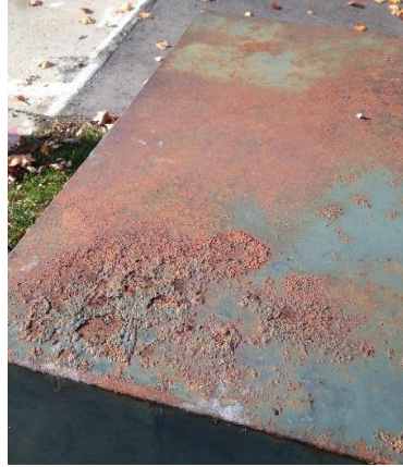
Figure 14: Padmounted Transformer with Surface Corrosion
