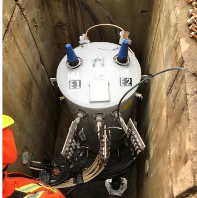
4 Figure 2: Submersible Vault
