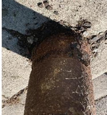
4 Figure 5: Corrosion on Steel Pole Base
