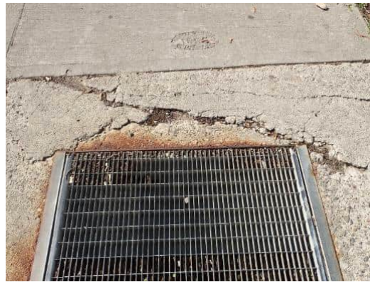
9 Figure 23: URD Vault with Deficient Roof
