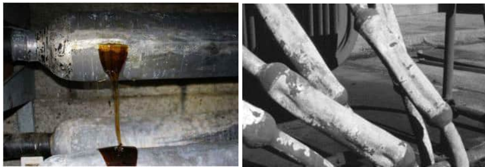
12 Figure 4: Sample PILC Joint with a Split Sleeve, i.e. Leaker (Left) and Collapsed Cable Splice (Right)
