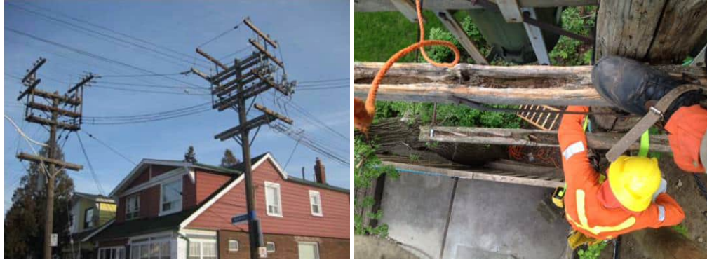
1 Figure 8: Box Construction (left). Replacing a transformer on a 2 poor condition Rear Lot pole (right)
