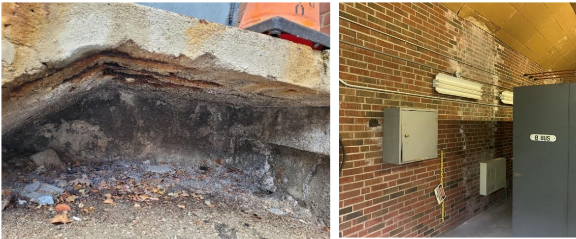
11 Figure 8: Examples of architectural deterioration at stations, from left to right: George and Duke 12 Station deteriorated concrete stairs, Centre Drive Station water infiltration from roof.
