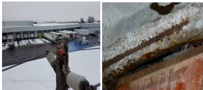
16 Figure 4: Pole fire caused by Tracking (left), Exposed and rusted rebar in Network Vault (right)
