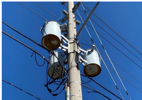
9 Figure 7: Rusted Overhead Transformers at Risk of Leaking Oil
