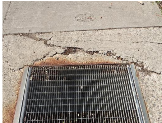
9 Figure 23: URD Vault with Deficient Roof
