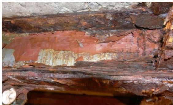
6 Figure 8: Corroded I-beams
