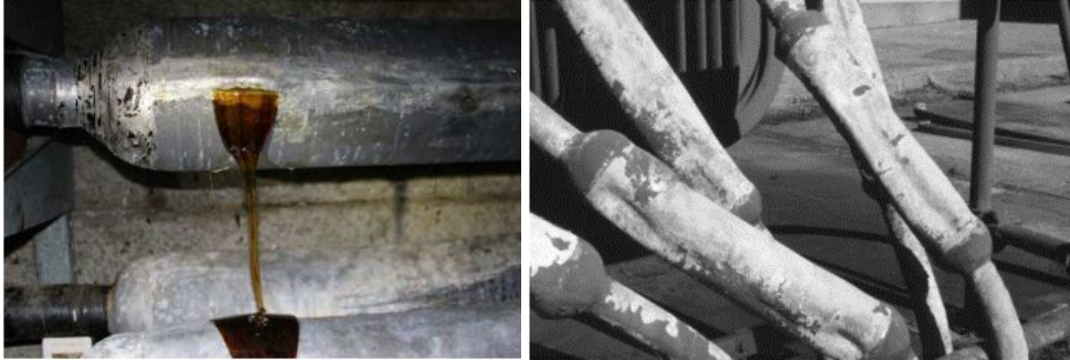
12 Figure 4: Sample PILC Joint with a Split Sleeve, i.e. Leaker (Left) and Collapsed Cable Splice (Right)
