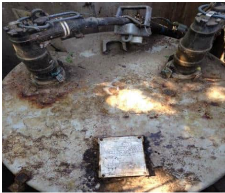
8 Figure 10: Corrosion on top of a Submersible Transformer
