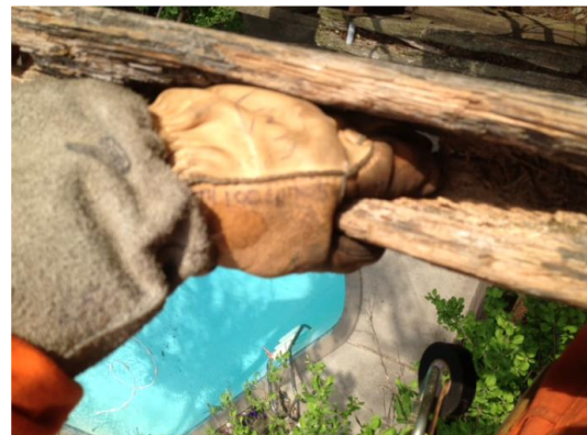
14 Figure 7b: Poor condition pole in close 15 proximity to swimming pool
