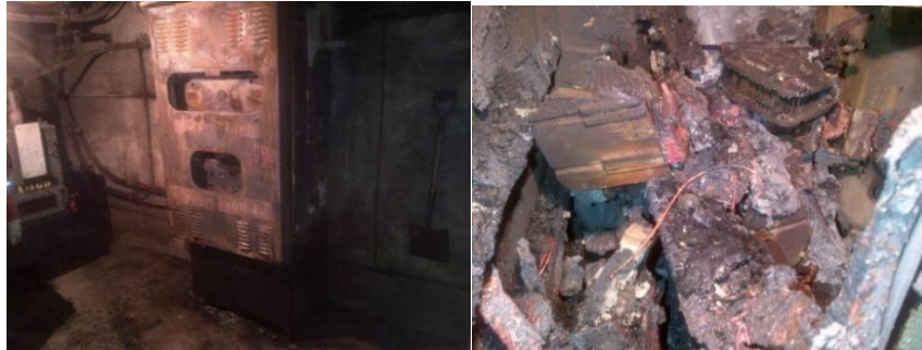
3 Figure 12: Damage from a network vault fire
