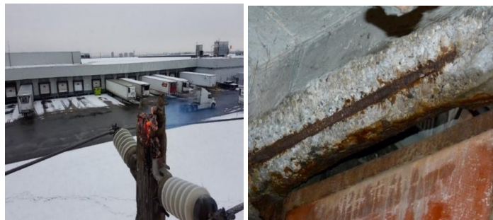
16 Figure 4: Pole fire caused by Tracking (left), Exposed and rusted rebar in Network Vault (right)
