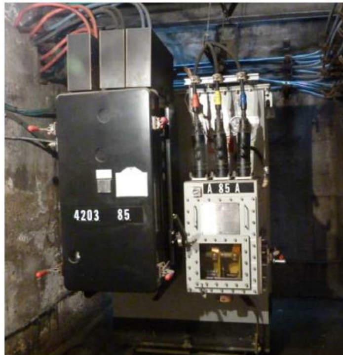
11 Figure 7: An Example 500 kVA Network Unit
