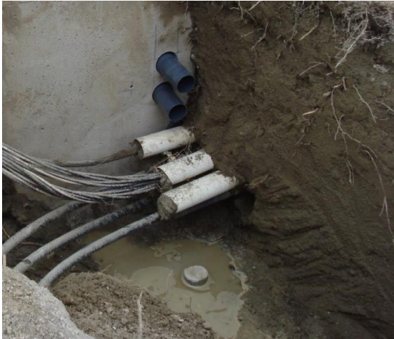
Figure 4: Clogged PVC Ducts
