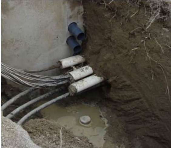
Figure 4: Clogged PVC Ducts
