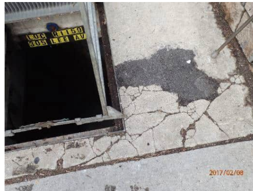
10 Figure 24: URD Vault Deficient Roof Temporarily Repaired with Asphalt
