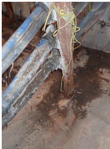
8 Figure 28: Example of Switch Supports that have rusted
