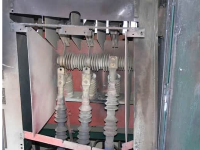
3 Figure 21: Padmounted switch with contaminant build-up
