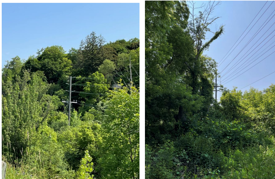
6 Figure 31: Difficult-to-Access Overhead Circuits on Humber River across Kipling Avenue
