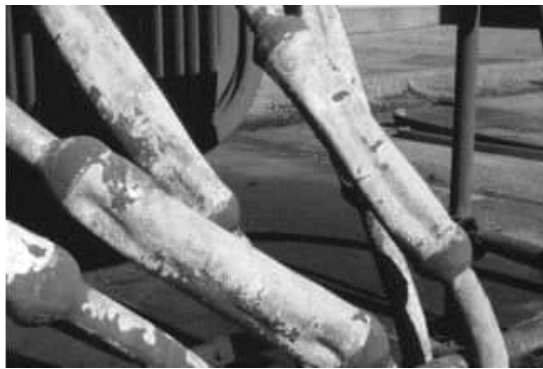
11 Figure 9: Collapsed cable splice
