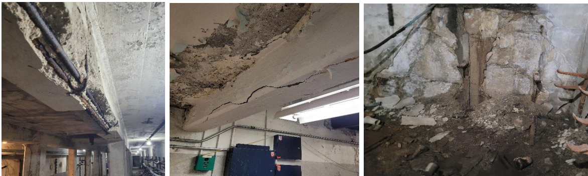
12 Figure 16: Examples of existing stations in critical condition, from left to right: George and Duke 13 Station, beam with exposed rebar, Defoe Station cracked beam, Junction Station deteriorated 14 foundation wall.
