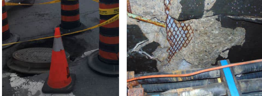
1 Figure 11: Cable Chamber roof in HI5 condition (left), Cable chamber roof inside view (right)
