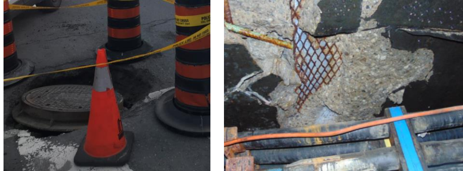
1 Figure 11: Cable Chamber roof in HI5 condition (left), Cable chamber roof inside view (right)
