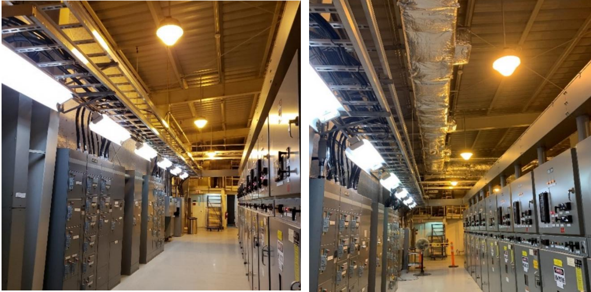
1 Figure 14: Examples of HVAC additions at Stations: Cavanagh Station without additional air 2 conditioning (left) and after with ducts and venting installed for keeping air temperature and 3 equipment cool (right).
