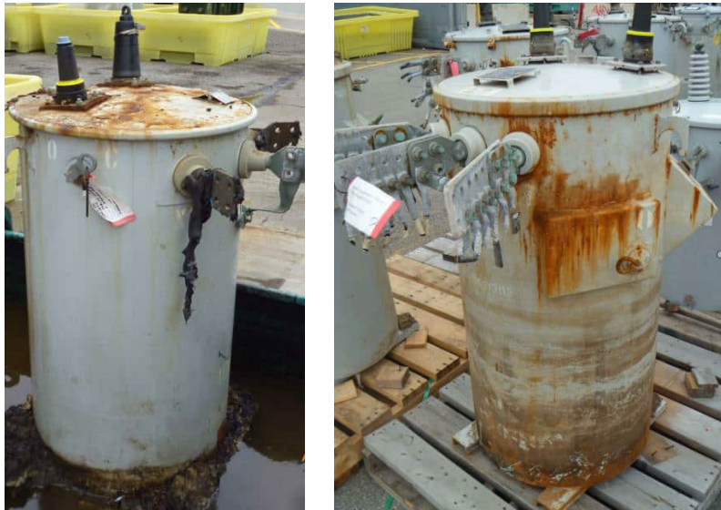
14 Figure 13: Mild steel single-phase submersible transformers with heavy corrosion
