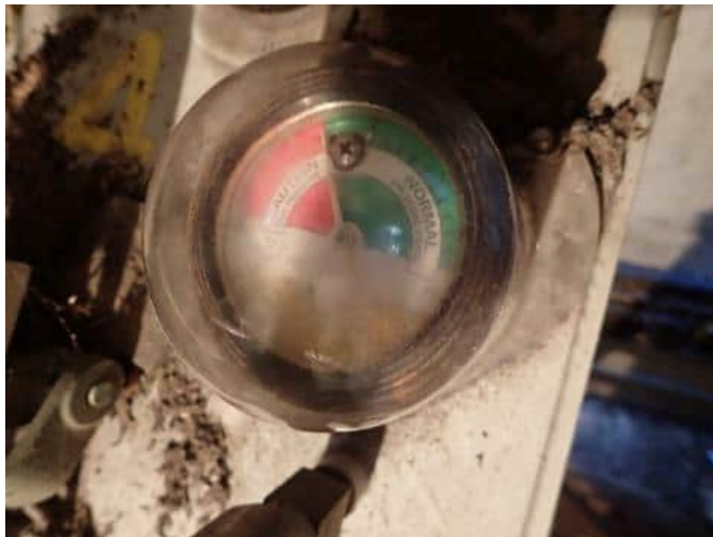
16 Figure 27: Example of a SF6 Switch with a “Low SF6” Reading
