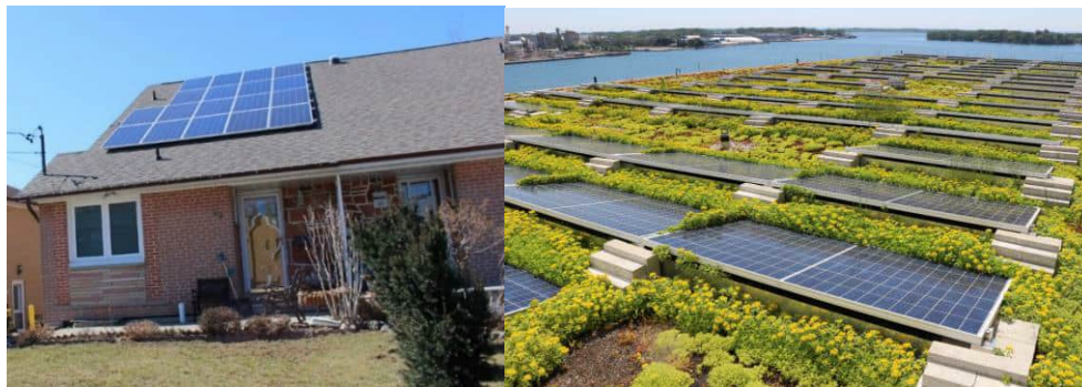
17 Figure 1: Residential (left) and Commercial (right) DER Installation
