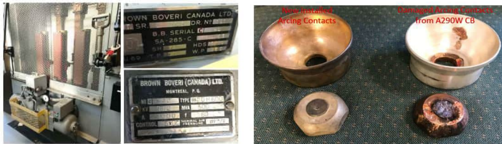
11 Figure 4: Failed Switchgear Air Blast breaker and damaged arcing contacts
