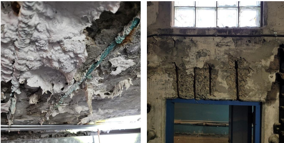
15 Figure 3: Examples of structural deterioration at stations, from left to right: Wiltshire Station 16 exposed and corroded rebar with significant water infiltration, Wiltshire Station exposed rebar in 17 concrete wall.
