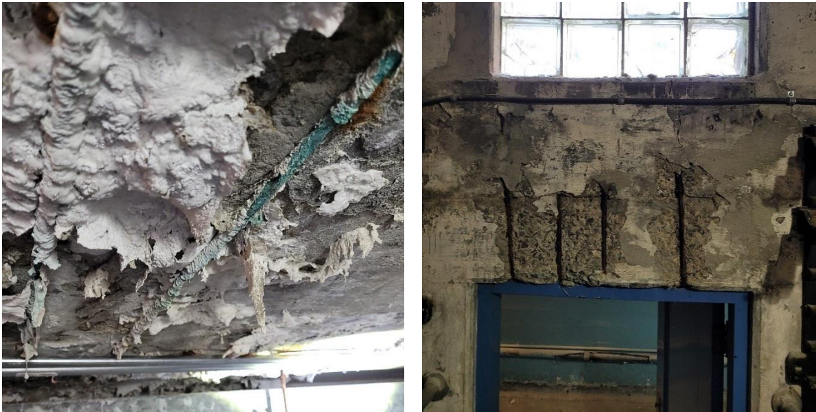
11 Figure 3: Examples of structural deterioration at stations, from left to right: Wiltshire Station 12 exposed and corroded rebar with significant water infiltration, Wiltshire Station exposed rebar in 13 concrete wall.
