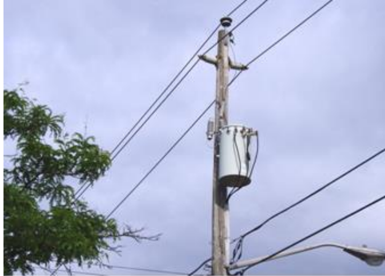
1 Figure 13: Overhead Distribution Transformer
