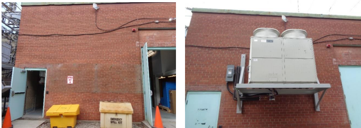
6 Figure 13: Examples of HVAC additions at Stations: Strachan Station without additional air 7 conditioning (left) and after with two new condensing units installed for keeping air temperature 8 and equipment cool (right).
