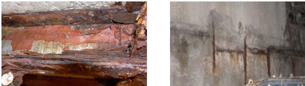
10 Figure 2: Underground vault structural deficiencies
