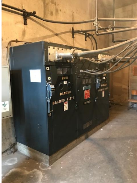
1 Figure 34: Example of Legacy Switchgear
