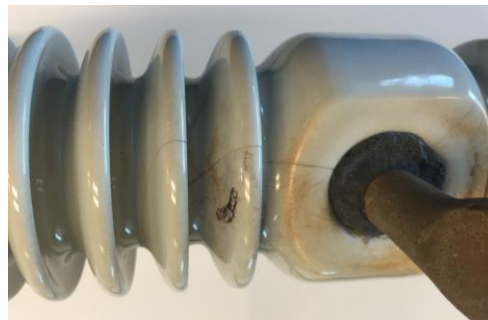
14 Figure 12: Porcelain insulator with small cracks in the shell and scorch marks
