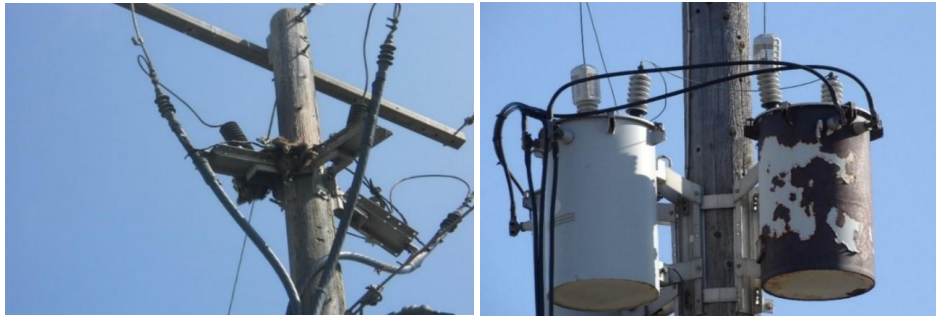
6 Figure 10: Animal Contact on Metal Switch Bracket (Left)/Rusted Overhead Transformers at Risk of 7 Leaking Oil (Right)
