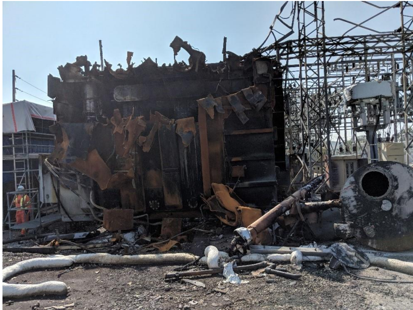
2 Figure 5: Post-Fire Damage at Finch Transformer Station Months Following a Major Event Day
