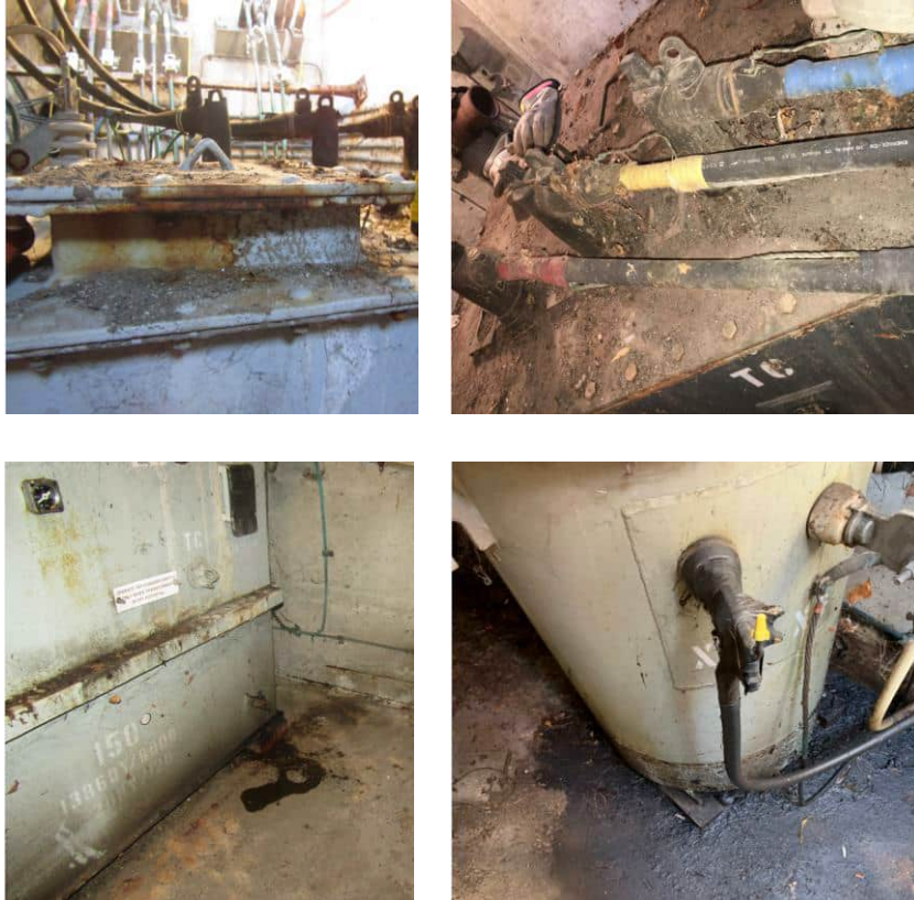
1 Figure 32: Examples of URD Transformers Exhibiting Corrosion on Lids and Oil Leaks
