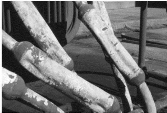
11 Figure 9: Collapsed cable splice
