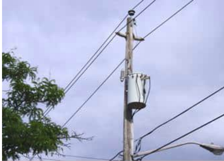
1 Figure 13: Overhead Distribution Transformer
