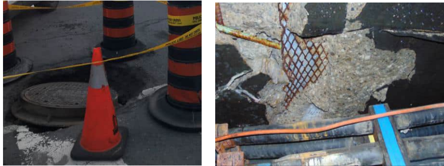
1 Figure 14: Cable Chamber Roof in HI5 Condition (Left), and Roof Inside View (Right)
