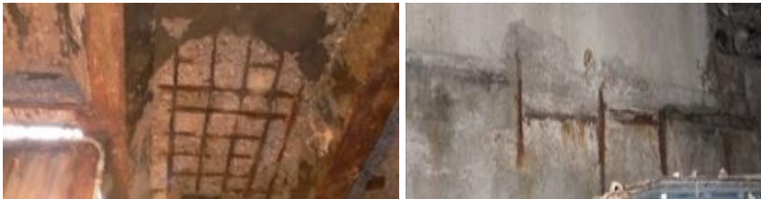
5 Figure 7: Roof and Wall with Exposed Rebar
