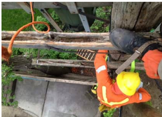
12 Figure 7a: Field crews replacing failed 13 transformer on pole in poor condition
