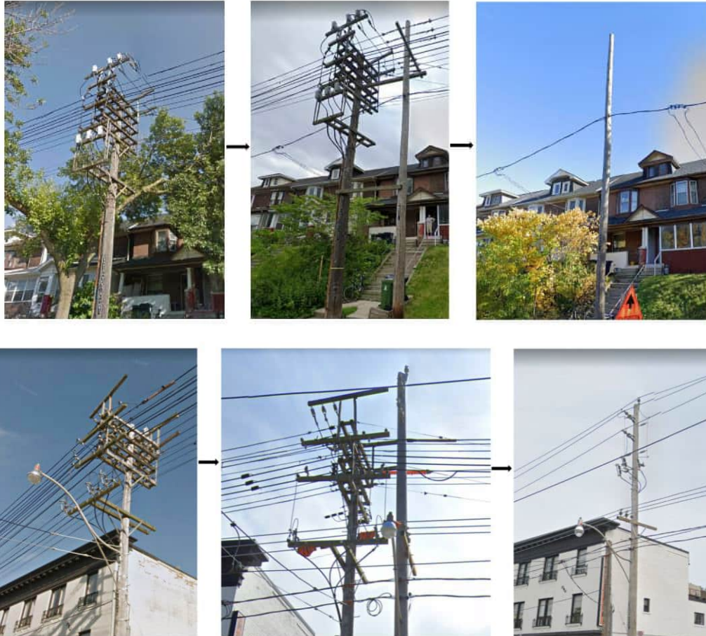
1 Figure 10: Actual box construction conversion project on Gerrard Street East at two locations. 2 Photographs on the left show 4.16 kV box construction poles prior to conversion. Photographs in 3 the middle are demonstrating the in-construction stage. The completed project is shown in the 4 photographs on the right, where all 4.16 kV box construction has been removed.
