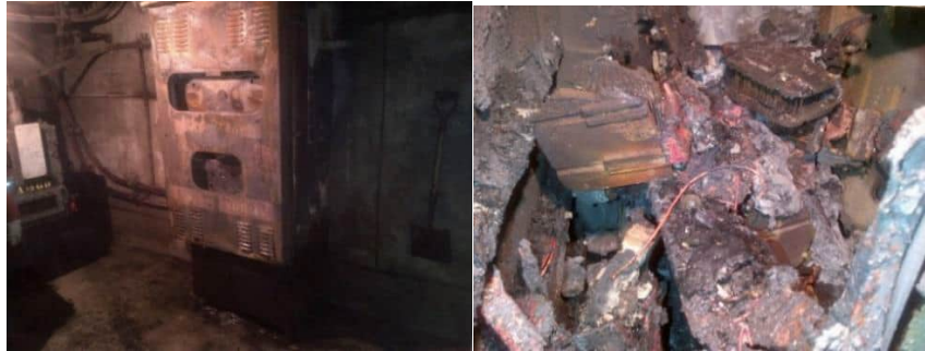
3 Figure 12: Damage from a network vault fire
