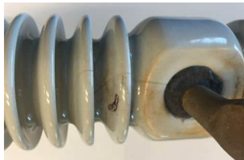
14 Figure 12: Porcelain insulator with small cracks in the shell and scorch marks
