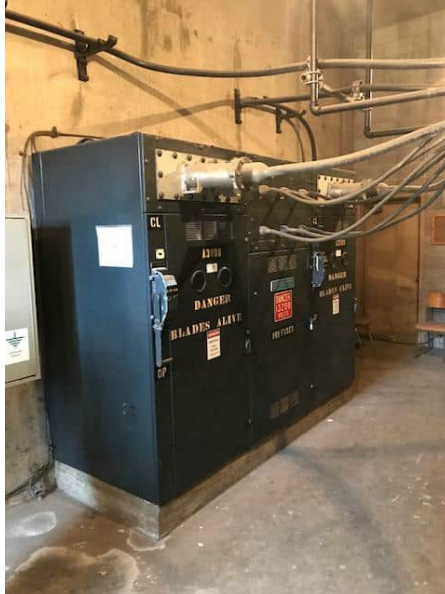
1 Figure 34: Example of Legacy Switchgear
