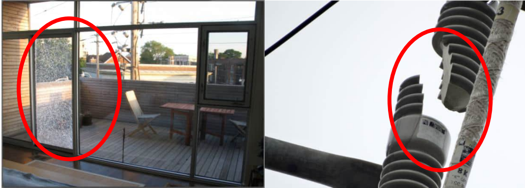
1 Figure 16: Porcelain Pothead Failure
