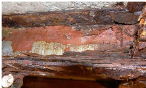
6 Figure 8: Corroded I-beams
