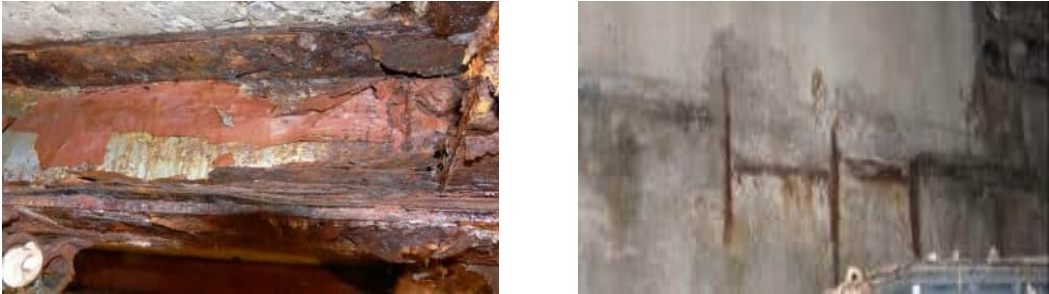
10 Figure 2: Underground vault structural deficiencies
