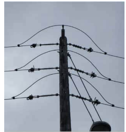
P11 (Existing Pole) – Overhead Conductors
