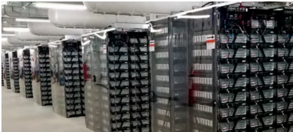
Renewable-enabling battery energy storage
