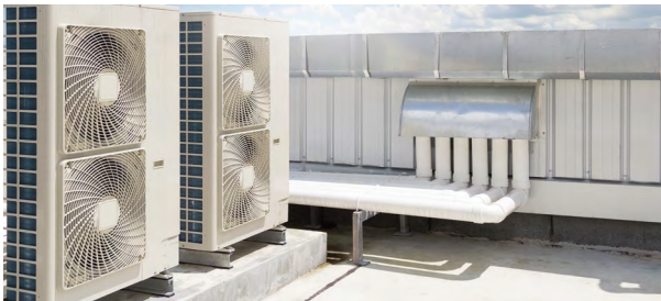
Heat pump field trial
