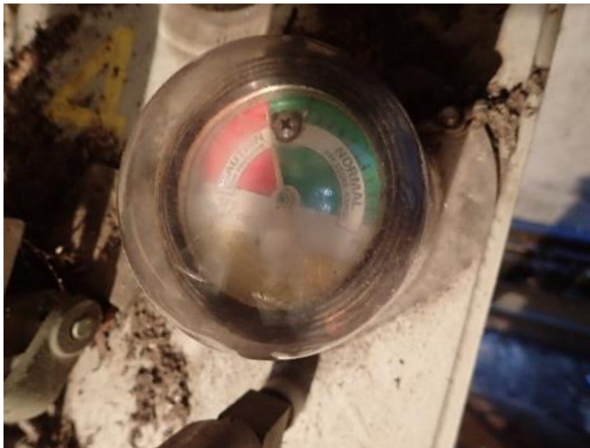
9 Figure 24: Example of a SF 6 Switch with a “Low” Reading
