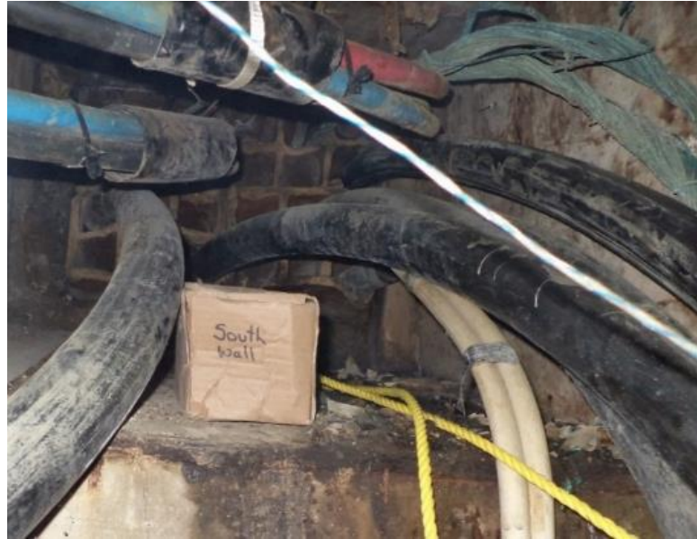
1 Figure 8: Example of a Legacy Square Clay Tile Duct
