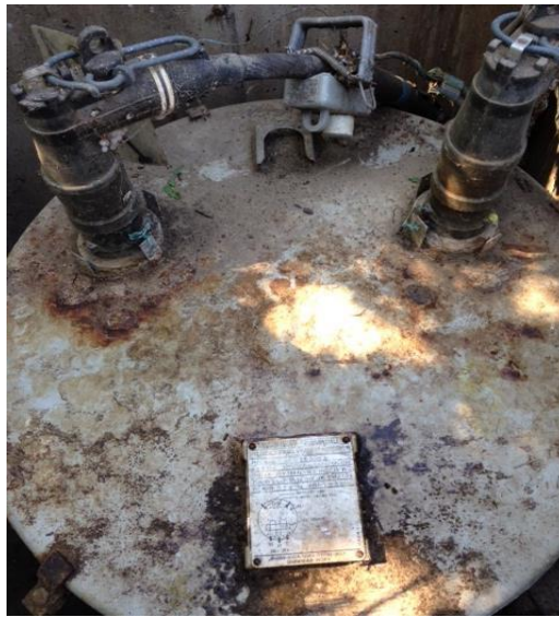
6 Figure 22: Corrosion on top of a Submersible Transformer
