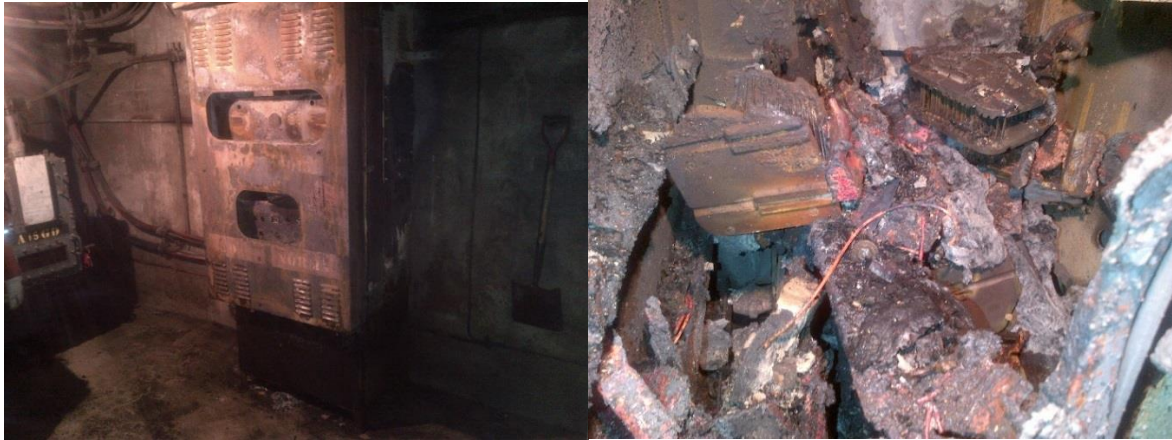
1 Figure 24: Damage from a network vault fire
