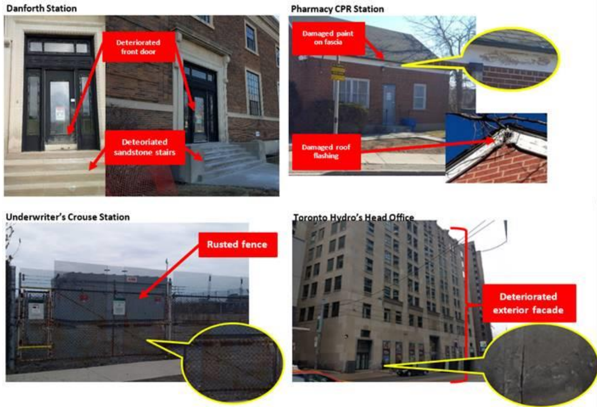
1 Figure 1: Examples of Toronto Hydro infrastructure that will be addressed through the Program
