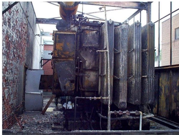
Figure 17: Failed Power Transformer TR2 at DuPont MS in 2003
