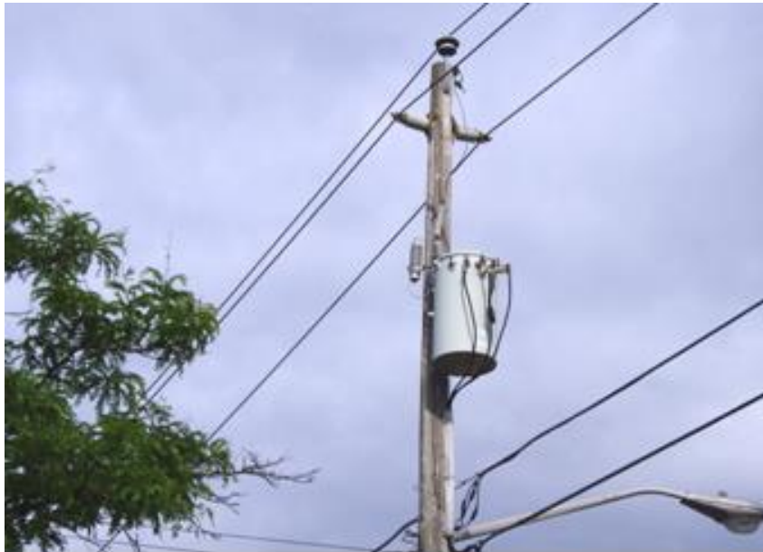
10 Figure 8: Overhead Distribution Transformer
