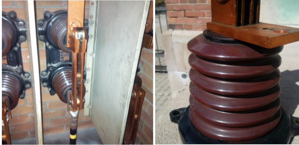
1 Figure 4: Failed Switchgear Insulator – Imperfection Difficult to Observe
