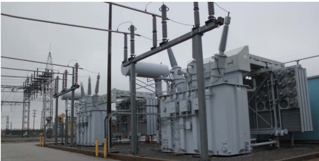
Figure 2-5 The Station Yard at Cavanagh Transmission Station
