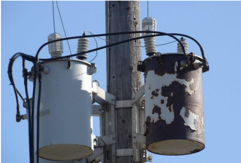
8 Figure 14: Rusted Overhead Transformers at Risk of Leaking Oil
