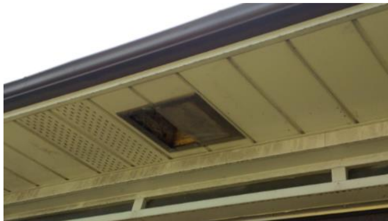
12 Figure 8: Damaged Exterior Light at Etobicoke Hartsdale Station
