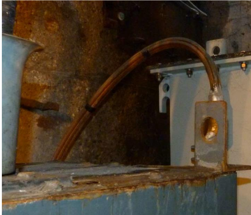
Figure 2: Rusting on Equipment Surface
