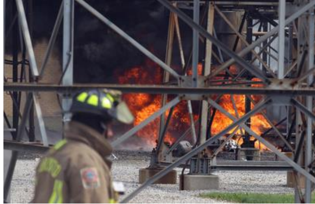
1 Figure 10: Catastrophic Failure of an Outdoor Circuit Breaker at Manby TS (Hydro One-owned)
