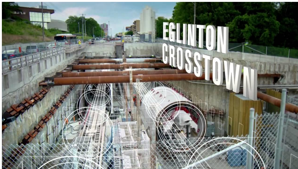
17 Figure 2: ECLRT Station Box
