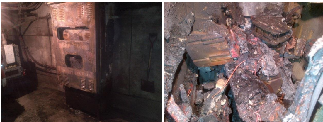
19 Figure 3: Damage from a Vault Fire Caused by Failure of an ATS Unit at 33 Princess Street on 20 January 16, 2012
