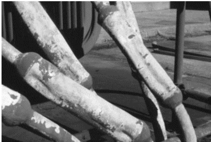
7 Figure 19: Collapsed cable splice
