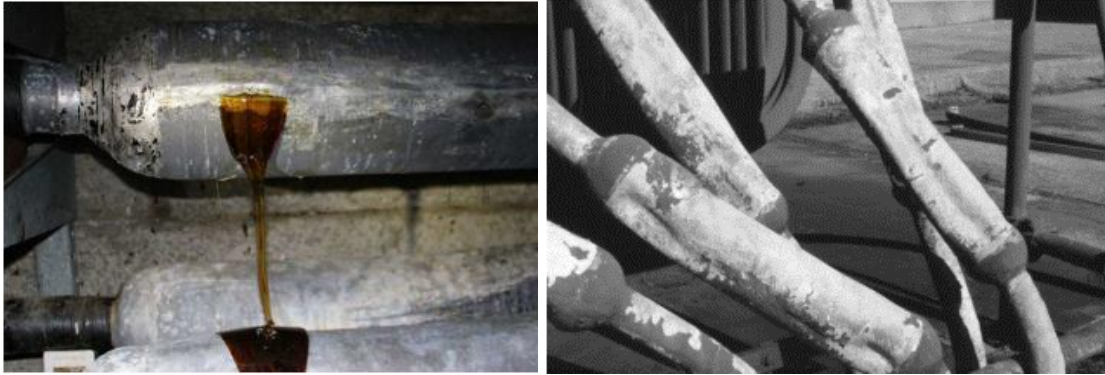
1 Figure 4: Sample PILC Joint with a Split Sleeve, i.e. Leaker (Left) and Collapsed Cable Splice (Right)
