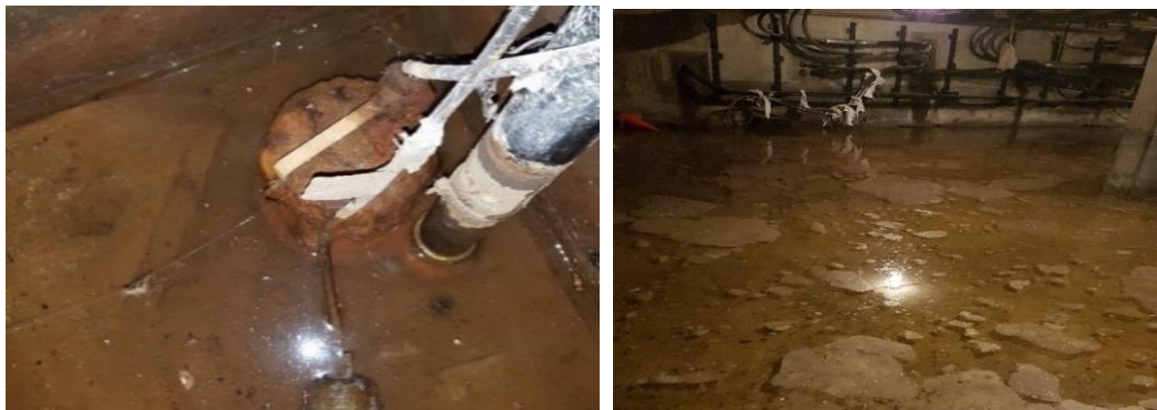
11 Figure 9: Heavily Corroded Sump Pump at Toronto Main Station (Left) and Dupont Station Flood 12 due to Sump Pump Failure in January 2018
