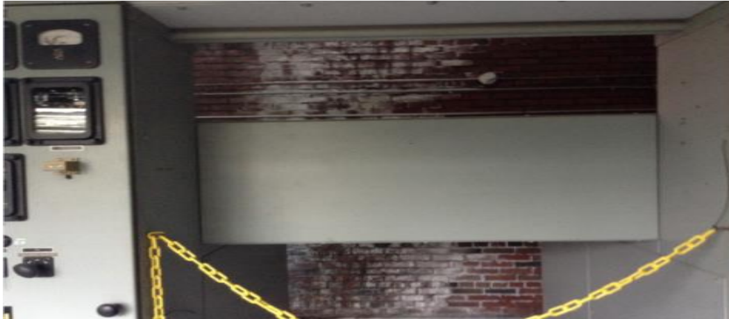
3 Figure 4: Damaged Wall at Etobicoke Neilson Drive Station
