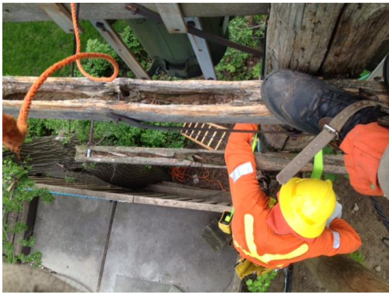
Figure 5: Field crews replacing failed transformer on pole in poor condition
