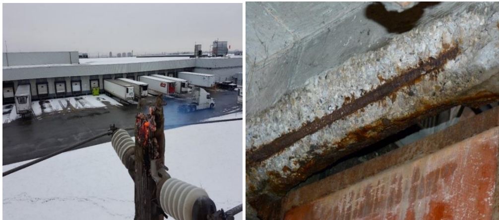
17 Figure 2: Pole fire caused by Tracking (left), exposed and rusted rebar in Network Vault (right)
