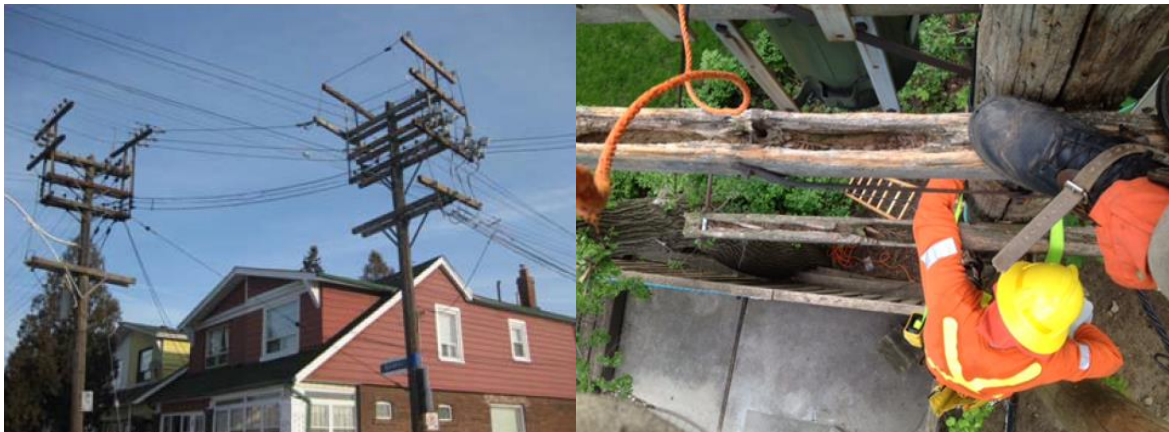
6 Figure 15: Box Construction (left). Replacing a transformer on a poor condition Rear Lot pole 7 (right)
