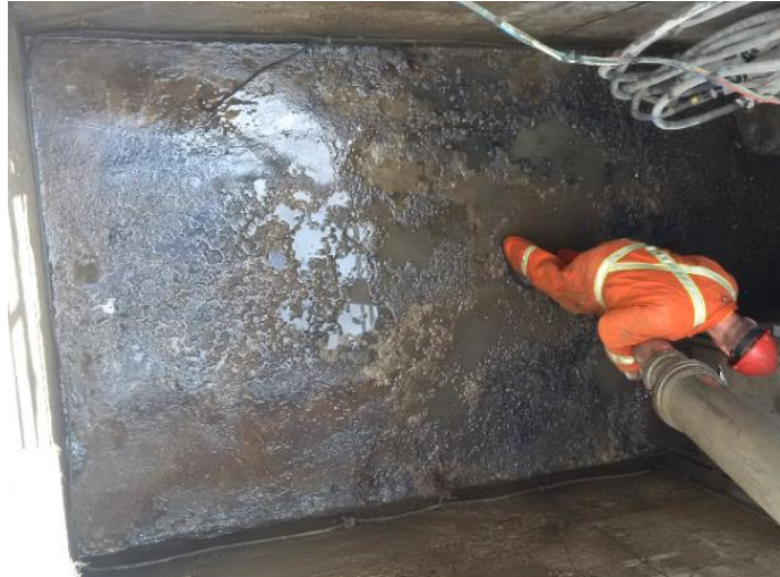
1 Figure 16: Deteriorated Vault Floor
