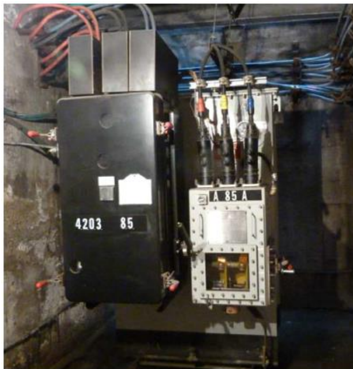
11 Figure 9: An Example 500 kVA Network Unit
