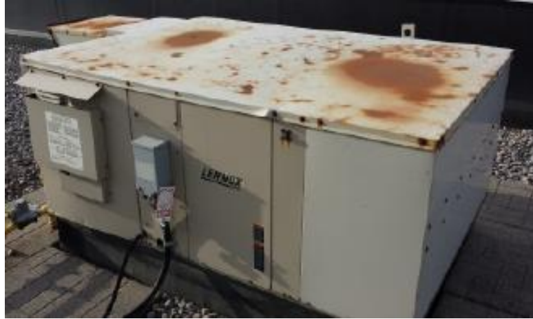
1 Figure 6: Rusted HVAC units at 500 Commissioners
