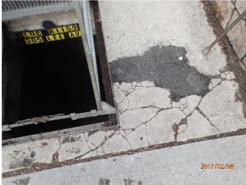
1 Figure 23: URD Vault Deficient Roof Temporarily Repaired with Asphalt
