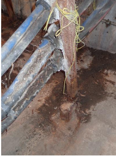
1 Figure 25: Example of Switch Supports that have rusted
