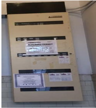
1 Figure 5: Cerberus Pyrotronics - Fire Panel at Carlaw Station
