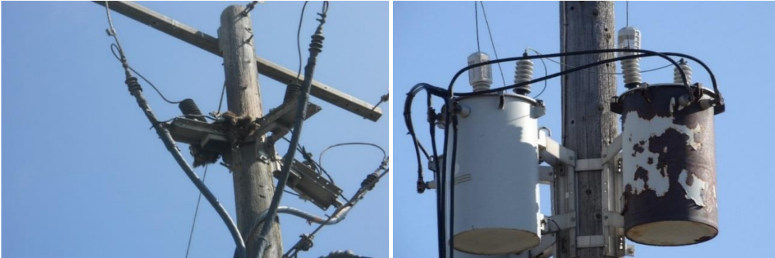
5 Figure 6: Rusted Overhead Transformers at Risk of Leaking Oil (Left)/Animal Contact on Metal 6 Switch Bracket (Right)
