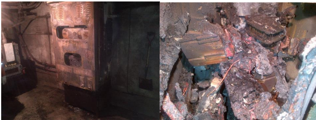
21 Figure 21: Damage from a Vault Fire caused by Failure of an ATS Unit
