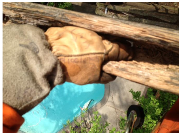
Figure 6: Poor condition pole in close proximity to swimming pool
