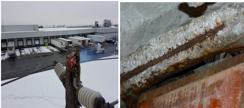
15 Figure 16: Examples of Reactive Work: Pole Fire Caused by Tracking (left), Exposed and 16 Rusted Rebar in Network Vault (right)
